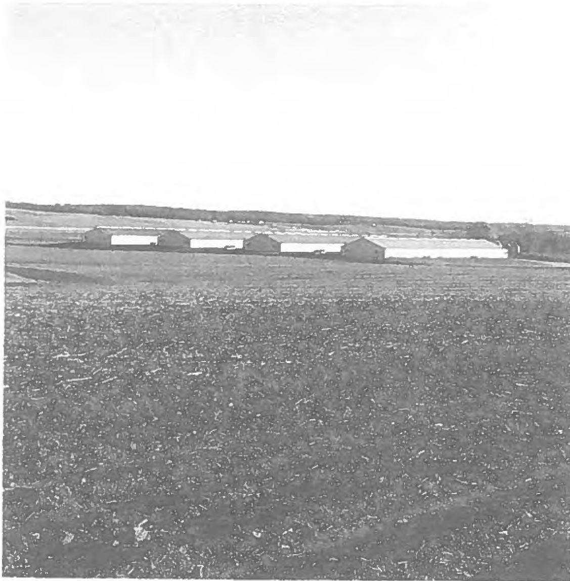
This is an expansion project of the outer two 1200 head swine barns over top of pollution control facilities
