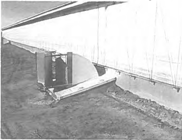
5. These pump-outs are covered with pit ventilation fans that are removed to agitate and load out livestock waste.
